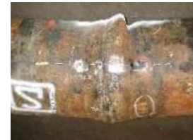
bent pipe joint with a lip
