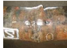
bent pipe joint with a lip
