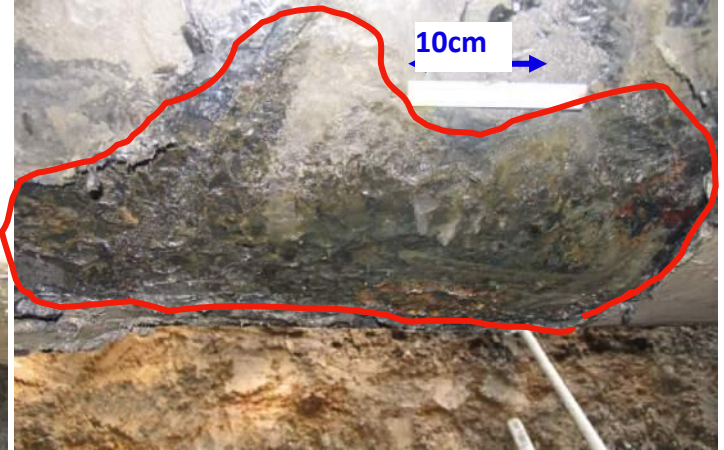
Corrosion due to disbonding
