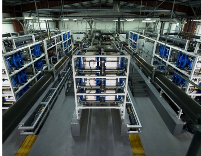
Vanadium Flow Battery Juices Onion Plant, POWER, https://www.powermag.com/vanadium-flow-battery-juices-onion-plant/
